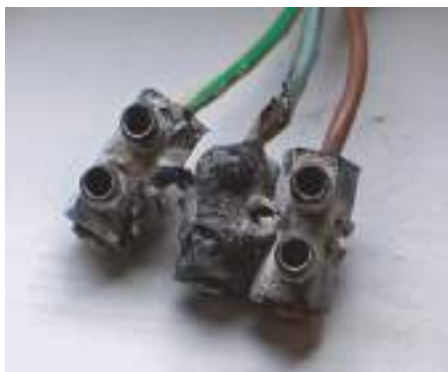
Fig. F84 Example of a carbonized connection
