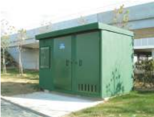
(a) Ground level walk in type substation
