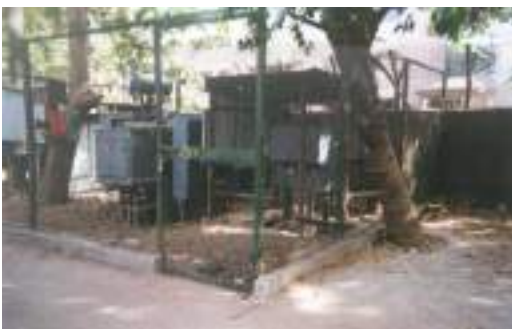
Fig. B53 Outdoor substation without enclosure
