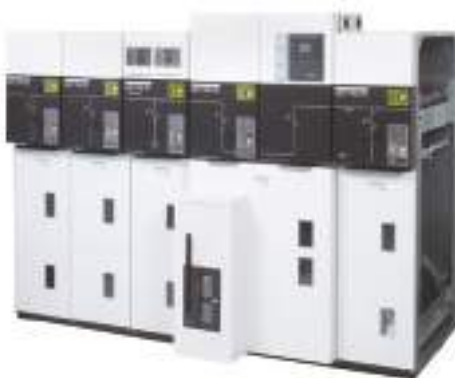
Fig. B35 Modular metal-enclosed switchgear
