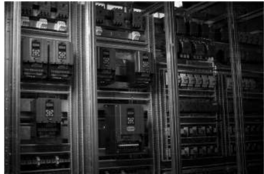
LV/ WTP PANEL 0.4 KV CCS TYPE
