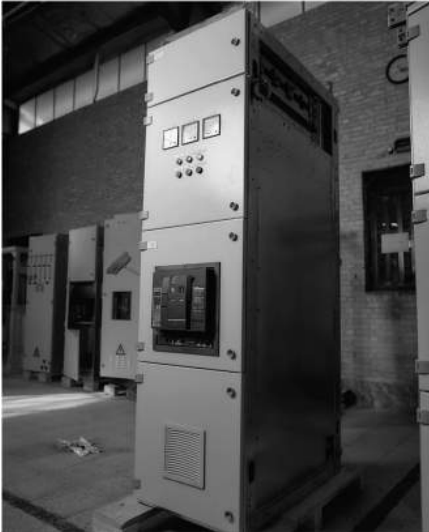
LV/ INCOMING PANEL 0.4 KV FCB TYPE
